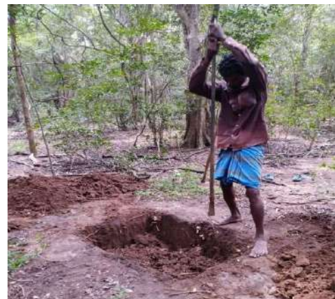
Figure 4-7: During Test pit excavation in tank bed of Pan kulam Aru Reservoir
