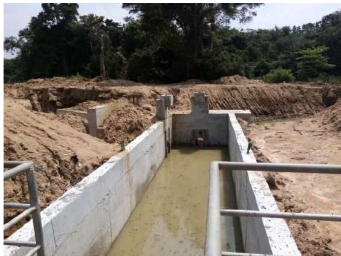
Figure 5-3: Issanwewa bifurcation structure
