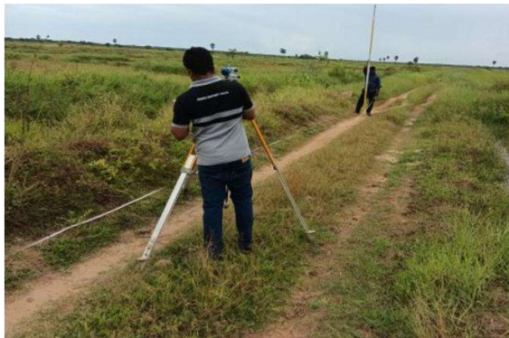
Figure 6-22: Improvement to FC8 farm road 0+000 to 0+250 in LB main channel in Kaddumurivu scheme in Rugam Division
