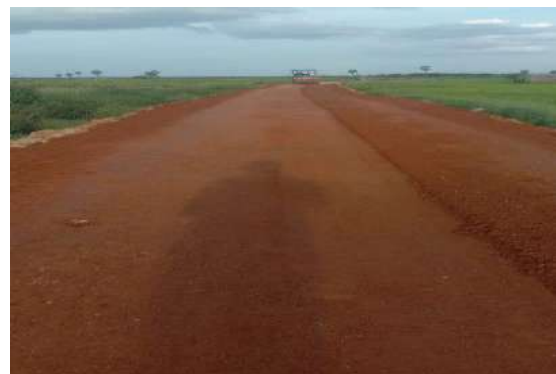
Figure 6-23: After construction of the FC8 farm road 0+000 to 0+250 in LB main channel in Kaddumurivu scheme in Rugam Division
