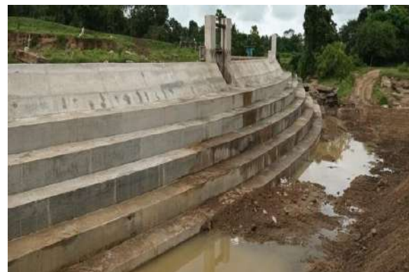
Figure 6-19: After Reconstruction of D/S spillway (LB) in Unnichchai tank in Unnichchai scheme in Rugam Division
