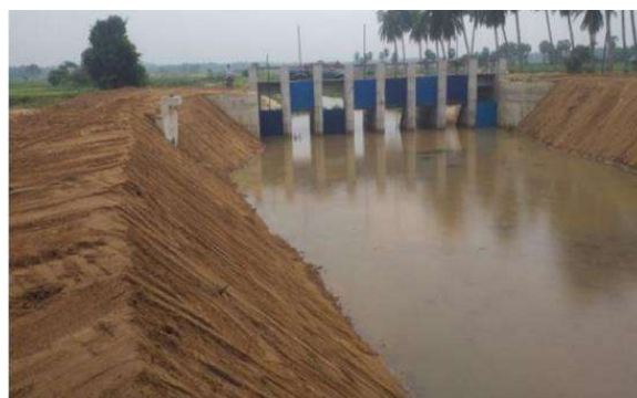
Figure 6-26: After Construction of Jeyapalan Anicut in Unnichchai scheme in Rugam Division, Batticaloa
