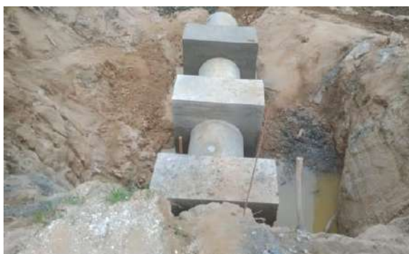
Figure 6-25: Repairs DR 02 morning glory spill in RB main channel stn 23+100 of Senanayaka Samudraya
