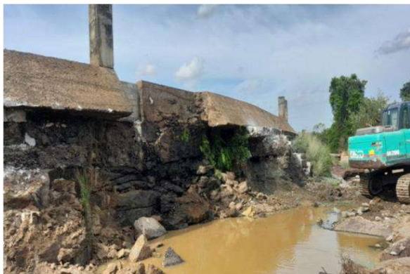
Figure 6-18: Before Reconstruction of D/S spillway (LB) in Unnichchai tank in Unnichchai scheme in Rugam Division
