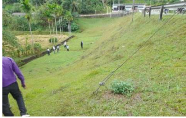
Figure 6-30: Inspection of seepages and depressions in downstream of the Denagama Tank Matara Division
