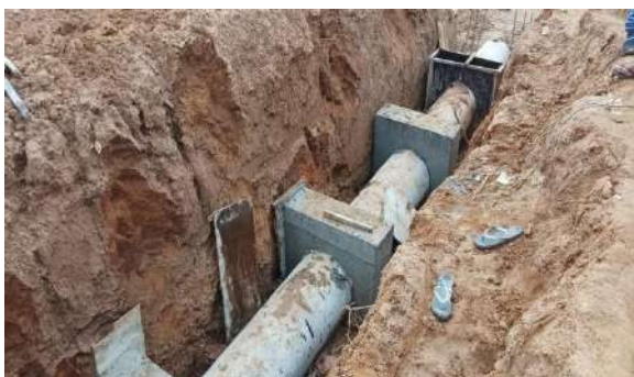
Figure 11-107: Construction of new canal for Bebiyawewa Tank to Meegas wewa tank from stn.0+000 to stn. 1+560
