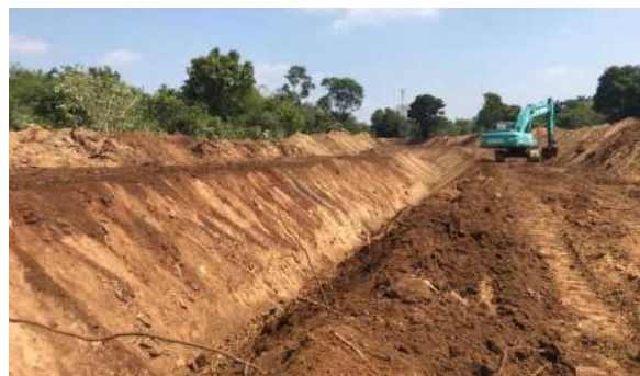
Figure 11-108: construction of new canal for Bebiyawewa Tank to Meegas wewa tank from stn.0+000 to stn. 1+560
