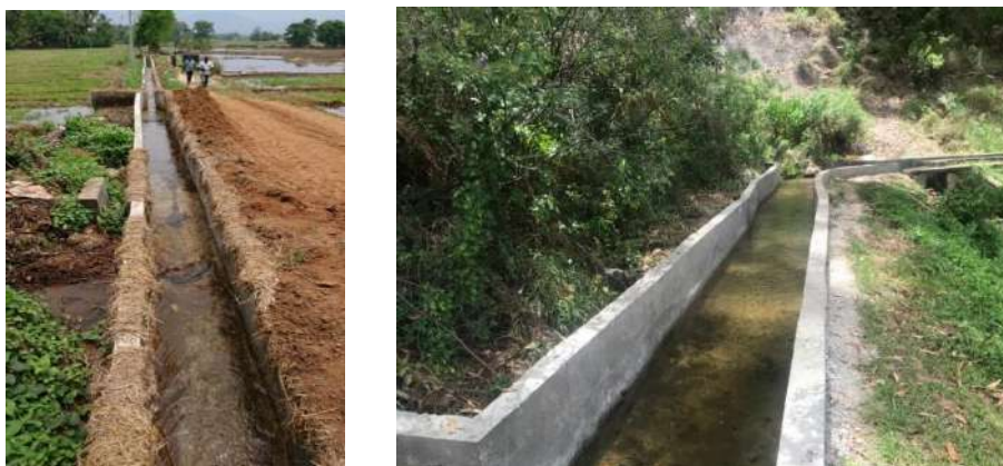
Figure 11-26: Construction of canal lining at 0+970 of main canal in Maha Eliya scheme
