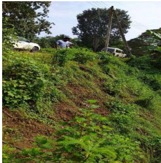
Figure12-4: Proposed location (temporarily filled breach) for the canal spill in Bathalagoda Feeder Canal
