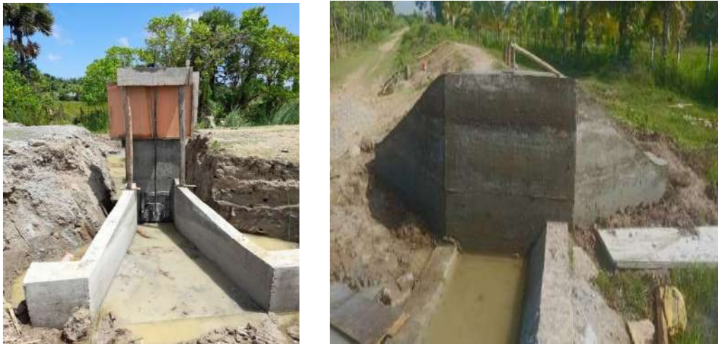
Figure 11-113: Construction of sluice and Improvement of spill in Wattukaweli in Puttalam Division
