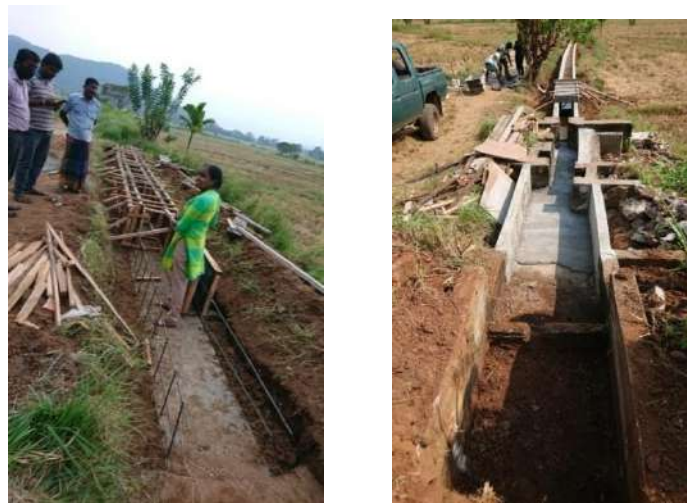
Figure 11-25: Construction of 40m long canal lining at RBMC FC 07 in Mapakadawewa scheme
