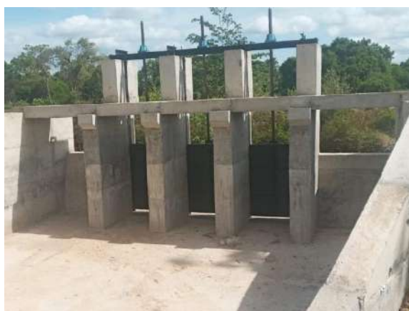
Spill gates of Walanthaliyawa Tank
