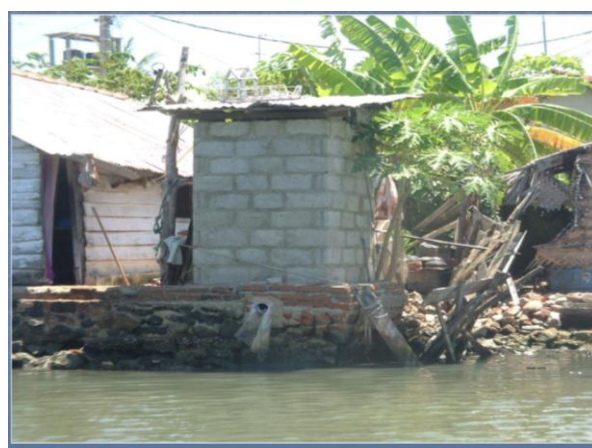
Figure 6 : Disposal of Raw Sewage to River Flows
